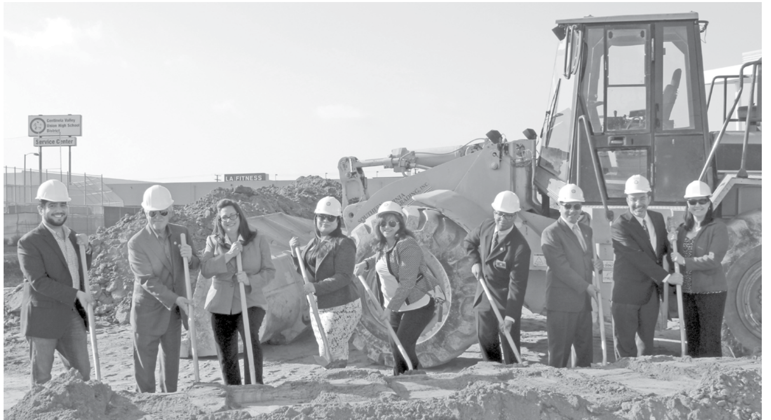
Lawndale High School broke ground this week on a two-story, 42,000 square foot building which will open during the 2016-17 school year. The building will house a student union, cafeteria, nine classrooms, and a computer lab. Pictured at the groundbreaking event are (L-R): John Vargas, El Camino Board Member, Jan Vogel, South Bay Workforce Investment Board CEO, Gloria Ramos and Maritza Molina, CVUHSD Board Members, John Gardner, Los Angeles Sheriff's Department Security Assistant, Hugo Rojas, CVUHSD Board President, Dr. Gregory O'Brien, CVUHSD Superintendent and Paula Rodas, Lawndale High School Principal. Photo courtesy of Centinela Valley Union High School District.
