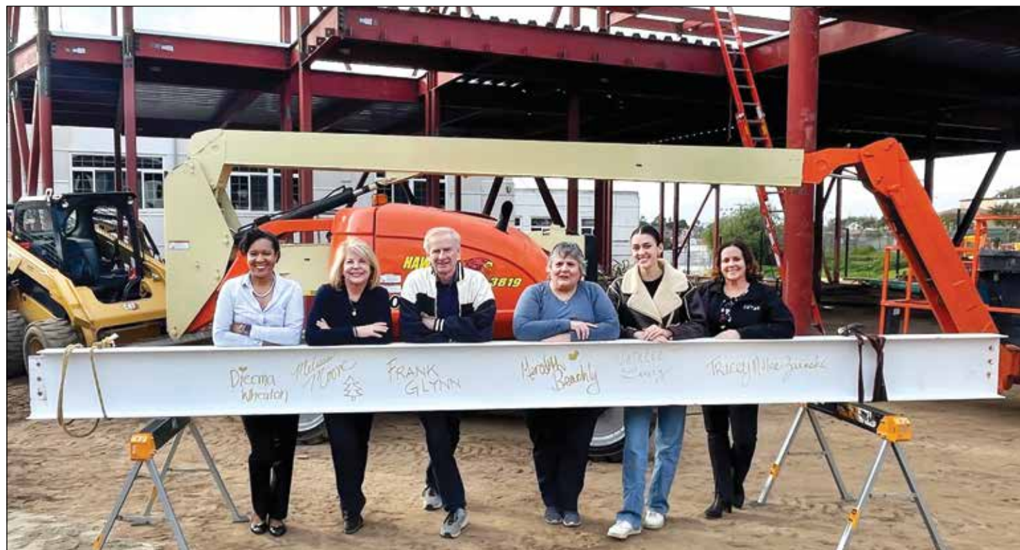
On February 3, El Segundo Unified School District hosted a topping ceremony for the new classroom building at Richmond Street School. A topping ceremony signifies the safe completion of the framing of the structure and a wish for continued good luck for the future of the building project—and its eventual occupants, elementary students and faculty. The last steel beam raised is painted white and is then signed by all the members of the ESUSD Governing Team, Facility Advisory Committee and Citizen Bond Oversight Committee members, Principal and Assistant Principal, erection crew, the building contractors, the architects, and other dignitaries. Photo provided by ESUSD.
